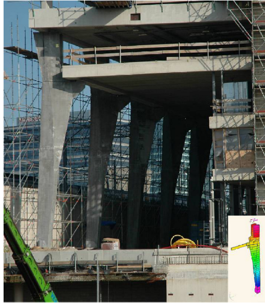
Figure 5. Column with narrow sharp concrete bracket.
